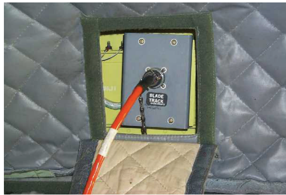
Figure 4. BLADE TRACK Bulkhead Receptacle Near STA 256
