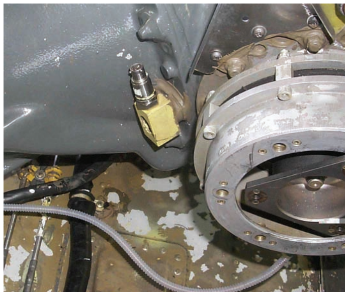
Figure 19. No. 2 Input Module Accelerometer Installation (ACC2)
